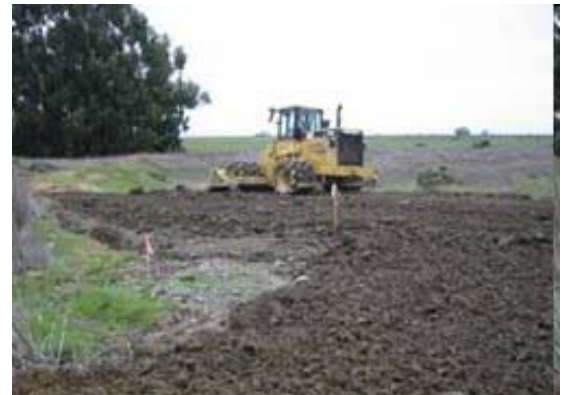
Work at the Hamilton wetland restoration project near Novato, involving the former Air Force base property, is aided by the materials from the Port of Redwood City deepening project
